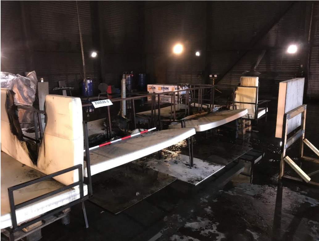
Damages on main fuel after test – test no 210526-1 – “below 1 nozzle”.
